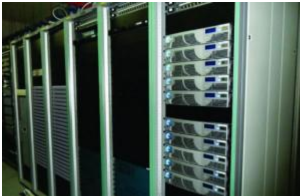
Isilon storage solutions at OSN.
