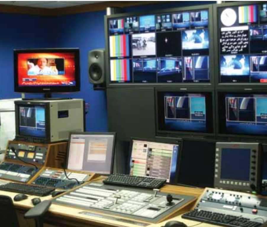
The control room at First Media.
